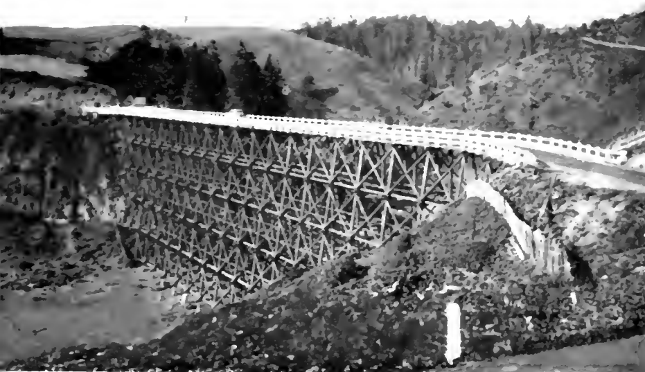
This is type of bridge on which loads are not now restricted, but must soon be because of continued deterioration
